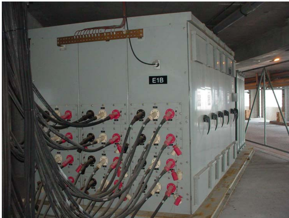
Figure 13-6. Newer Double-Deck Pier Switchgear
